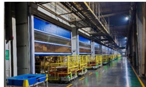
Environmental Protection Facilities at Hubei Linglong
