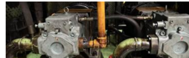
Hydraulic Station Motor Transformation
